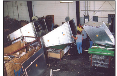
To date, the size and complexity of KoolDuct being fabricated in McDonald Air's shop is equal in versatility to that of conventional sheet metal ductwork.
